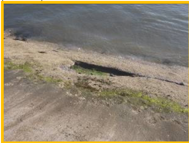
Cullercoates South Pier – locally poor defect on seaward sloping face (/4701C15)
