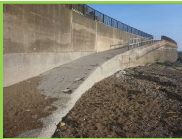
Brown's Bay access ramp with re-cast lower section (/4601C10)
