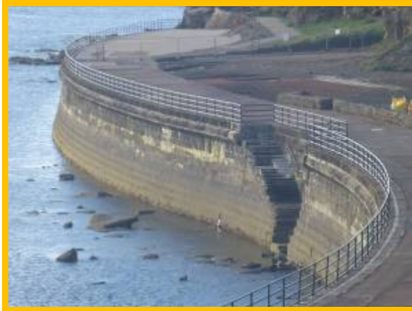
Stairwell which was infilled as part of the Southern Promenade Seawall Strengthening Scheme in 2020 (/4601C08) – photo from 2020 inspections
