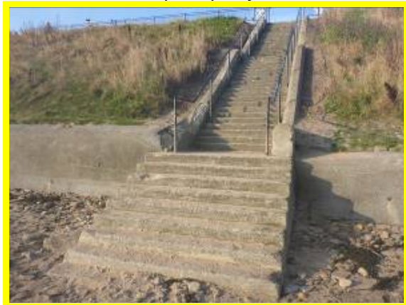
Abrasion damage at side-wall of beach access ramp (/4601C01)
