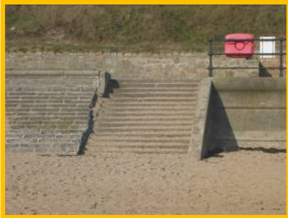
Damage at wing-wall of access steps (between /4701C18 and /4701C19) – locally poor
