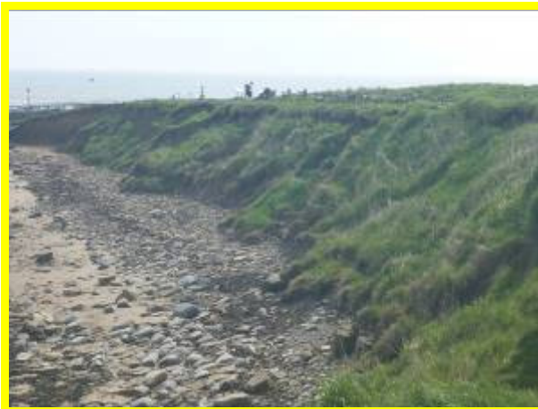
Erosion of soft earth slopes (/4401C25)
