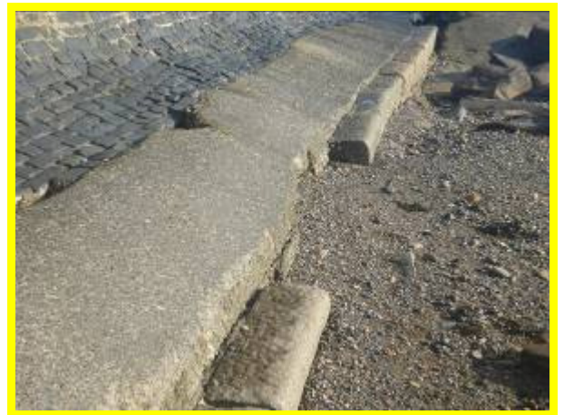
Some defects at the toe apron (/4701C06)
