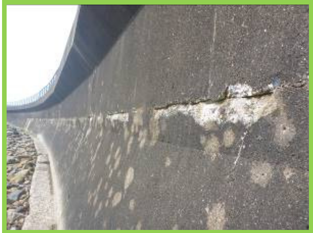
Trinity Road seawall in good overall condition but with some minor maintenance required on an ongoing basis (/4501C4)
