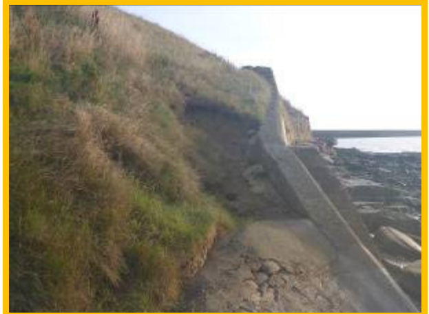
Erosion above wall (/4801C06)
