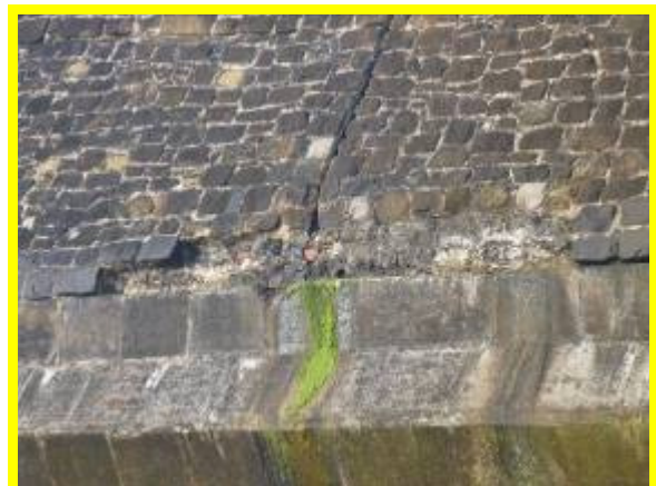
Missing brickwork (/4601C05) – from 2020 inspection
