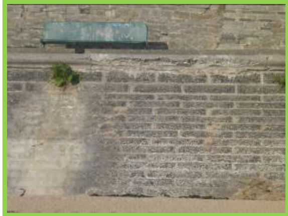
Abrasion to the revetment crest (/4701C19)
