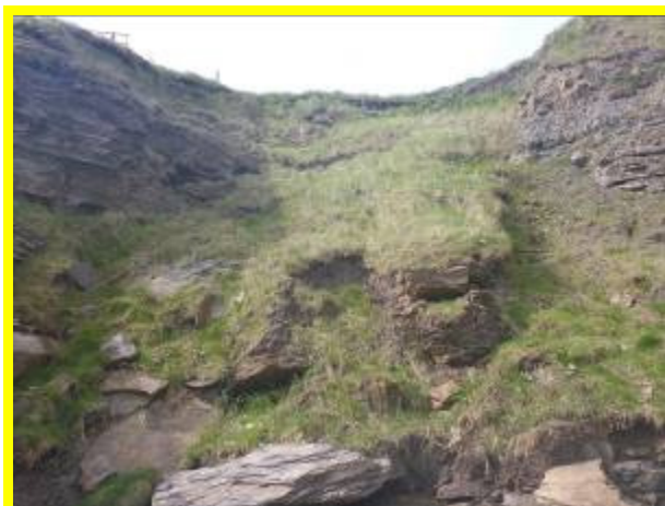
Remnants of 2009 slippage in soft material adjacent to Hartley Cove access steps (/4401C22)
