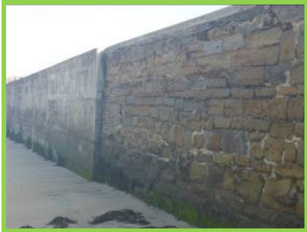
Cullercoates South Pier – vertical landward face showing original and encased sections (/4701C15)
