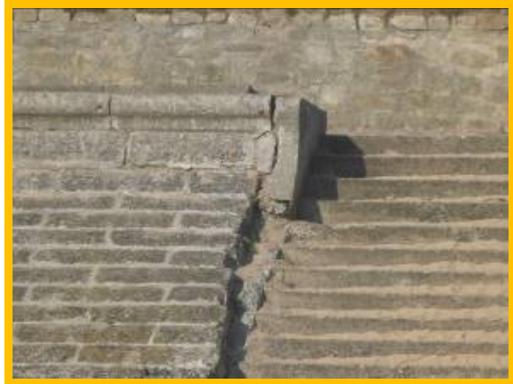
Damage at wing-wall of access steps (between /4701C18 and /4701C19) – locally poor
