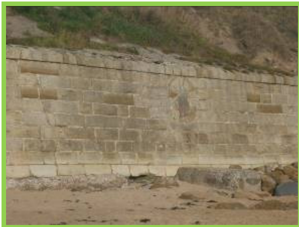
Undercutting and abrasion at toe of masonry tie-in wall (/4701C18)
