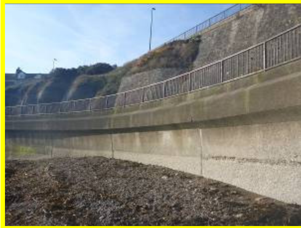
Brown's Bay southern sea wall in generally fair condition (/4701C01)
