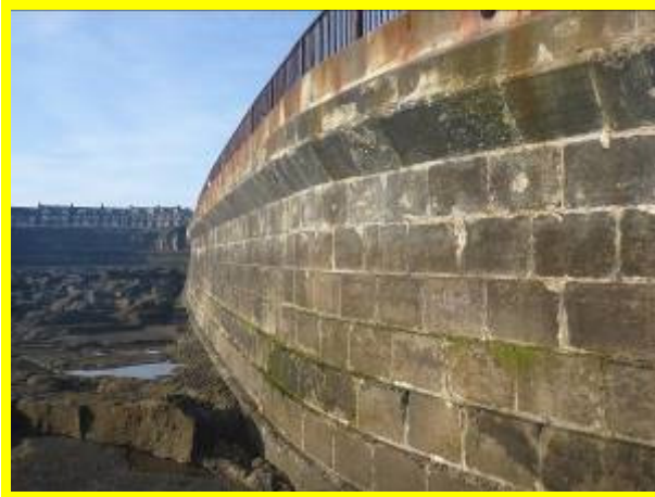
Brown's Bay northern sea wall in generally fair condition (/4601C10)
