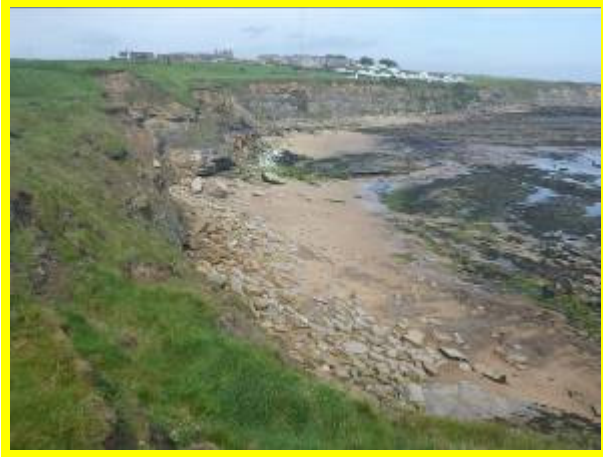
Slippages in soft material along upper cliffs and rock fall at base (/4401C22 & 24)
