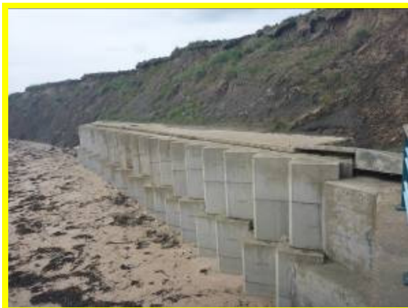
Uplifted deck above end of T-Block units at northern end (/4501C10)
