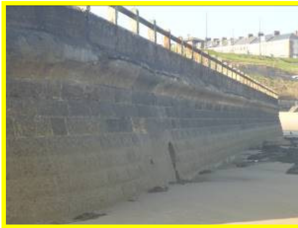
Wall abrasion at the Outdoor Pool (/4701C24)
