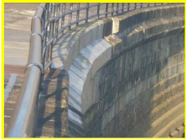
Repairs to wall as part of Southern Promenade Seawall Strengthening Scheme (/4601C08)
