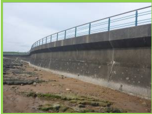
Trinity Road seawall in good overall condition, but with some minor maintenance required on an ongoing basis (/4501C04)
