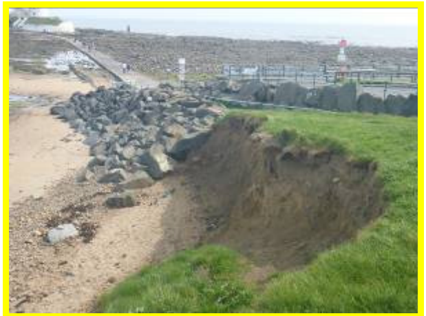
Erosion adjacent to rock revetment by St Mary's Island causeway (/4401C25)
