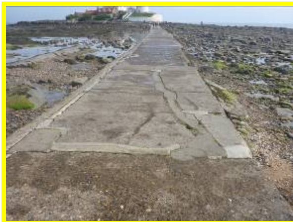
Partial loss of previous repairs to the causeway (/4401C25)
