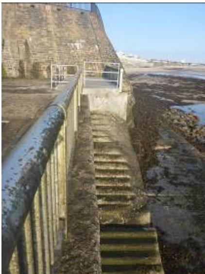
Closure of unsafe access steps along intermediate sea wall between Central and Southern Promenades (/4601C06)
