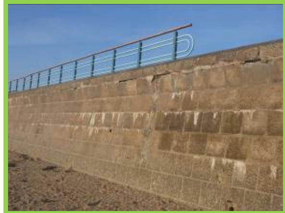
Previous repairs and local gaps in joints which would benefit from maintenance (/4501C07)
