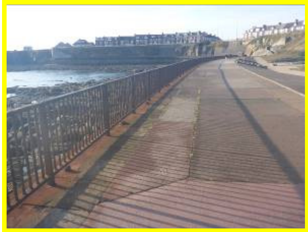
Minor surface cracks in promenade deck at northern end (/4601C10)
