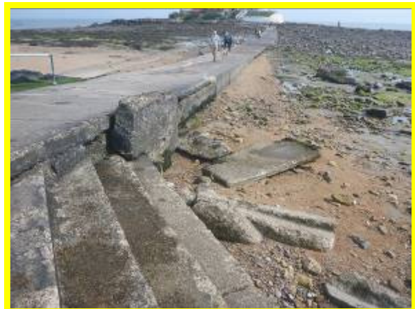
Concrete breaking-away from causeway edge (/4401C25)
