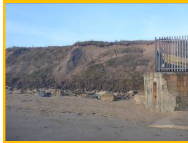
Slumping in cliffs to south of wall at boatyard (/4501C05)
