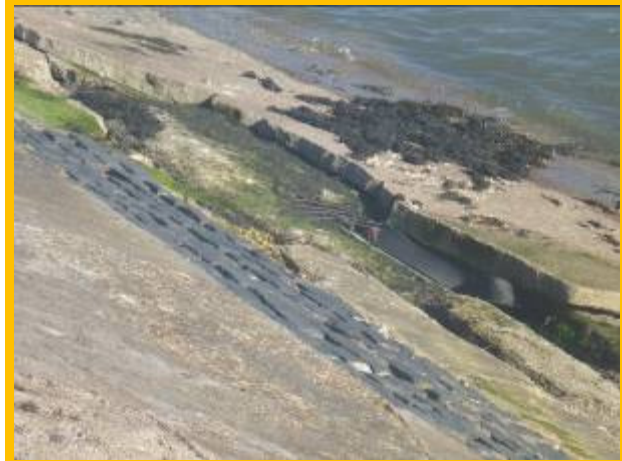
Damaged apron (/4701C27) – locally poor
