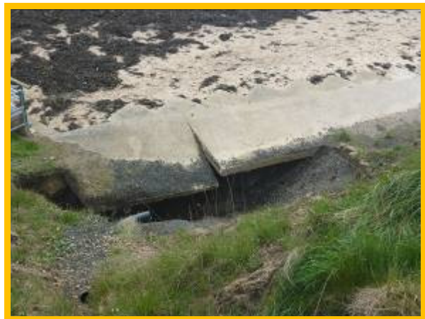
Voiding behind T-Block units at northern end (/4501C10)
