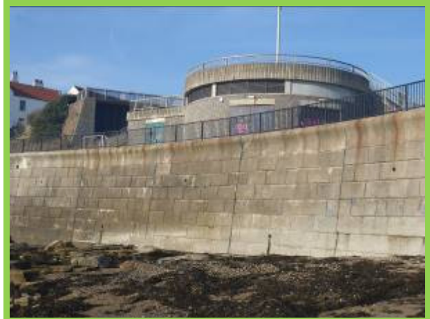
Middle section of sea wall in generally good condition but with face abrasion (/4701C05)
