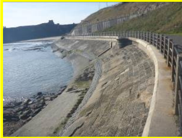
Sea wall in fair condition with damage and abrasion of the apron (/4701C27)
